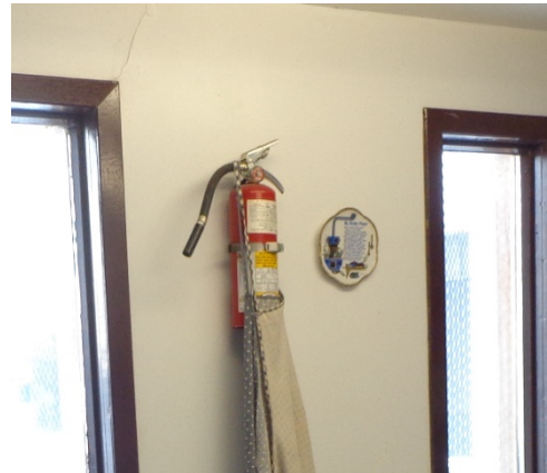
M6 – Typical fire extinguisher, missing inspection tag
