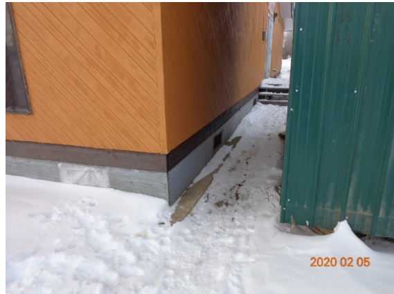
A10 – Plugged grilles into crawlspace
