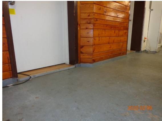
A28 – Floor elevation change (tripping hazard)
