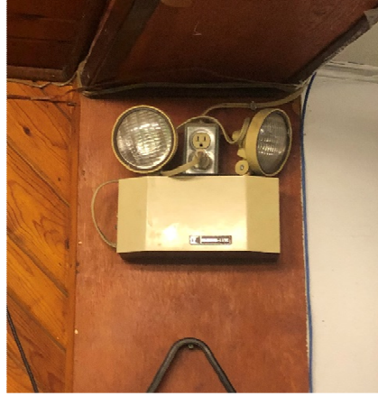
E8 – Emergency Light
