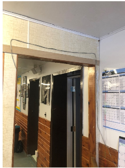
E4 – Exposed Telephone Wiring
