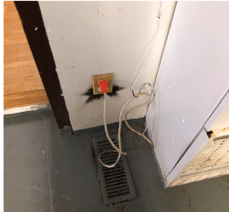
E2 – Electrical Outlet with Burn Marks
