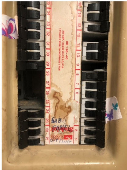
E3 – Main Distribution Panel
