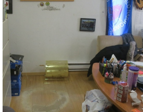
M2 – Typical office electric baseboard heater
