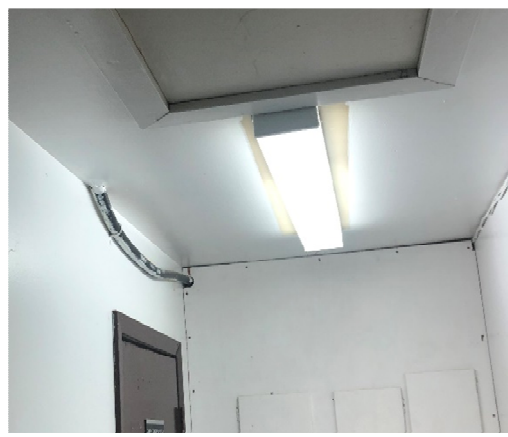
E6 – Fluorescent Light fixture
