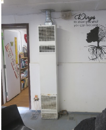
M1 – Propane furnace in main hall area.
