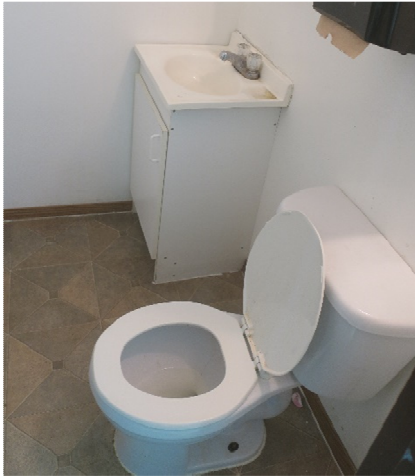
M3 – Public washroom toilet and vanity lavatory
